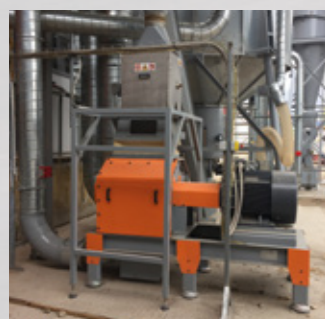
RP03 installato - installed.
